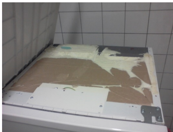
Figure 8: Missing diffusion barrier at the cabinet of appliance F01.
